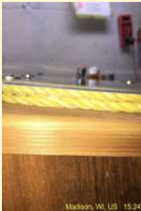
Side View Showing the Gap
